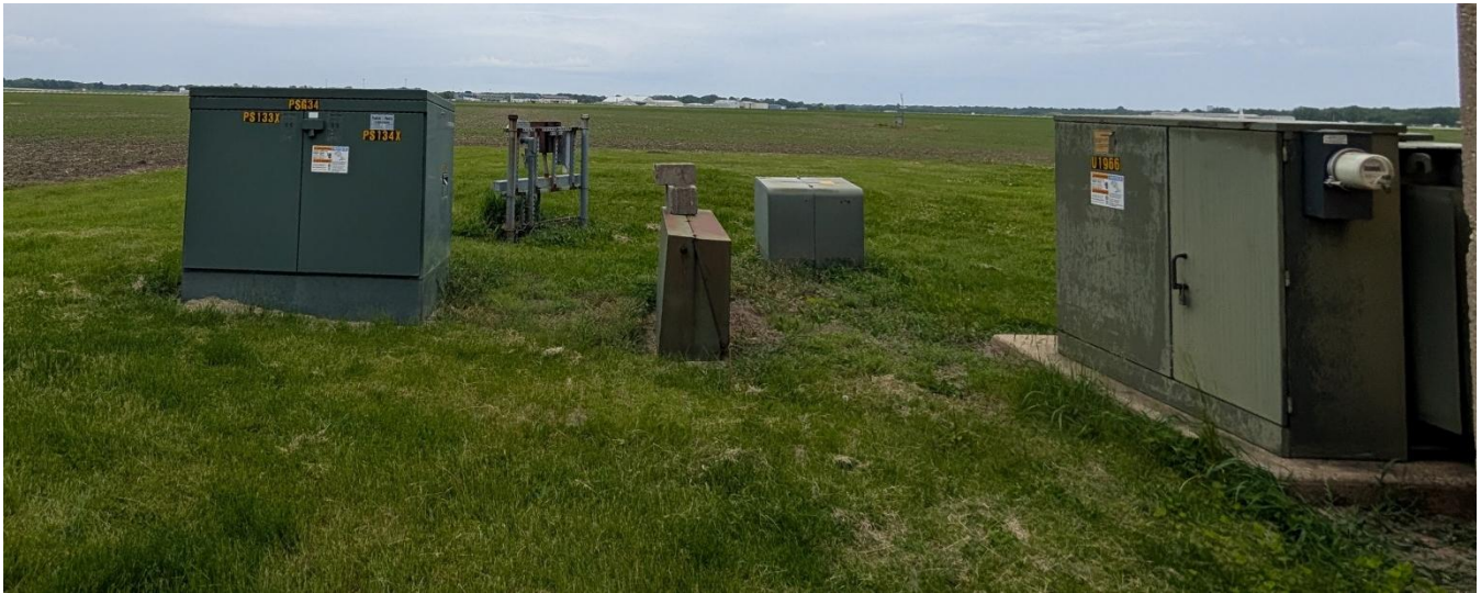
FIGURE C.3: U1966 FAA AIRFIELD LIGHTING VAULT
