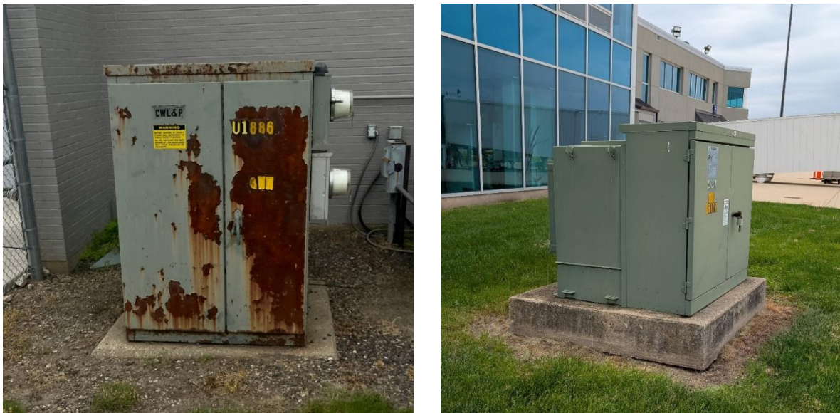
FIGURE C.2: AIRPORT TERMINAL TRANSFORMERS NORTH (U1886, LEFT) AND NORTHEAST (U6173, RIGHT)
