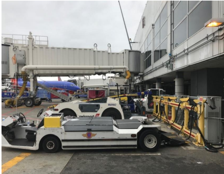
FIGURE 4.3 TYPICAL AIRPORT EGSE CHARGING STATION
