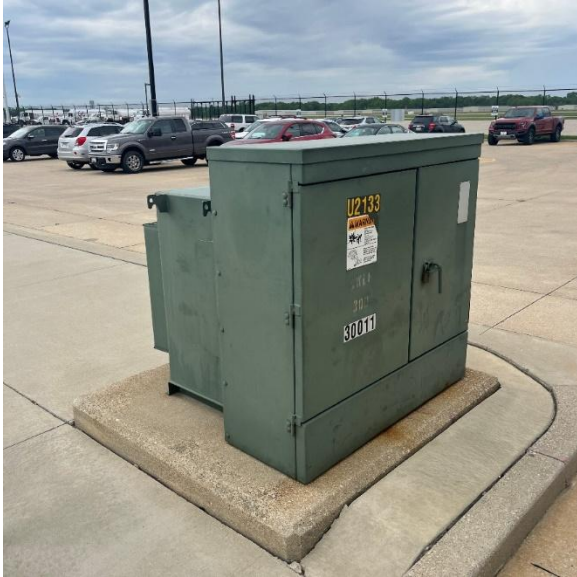
FIGURE C.1: AIRPORT TERMINAL SOUTH-SIDE TRANSFORMER
